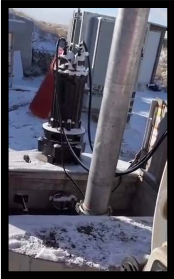
Picture of New Pump at Wagon Wheel Lift Station ready to be installed.
