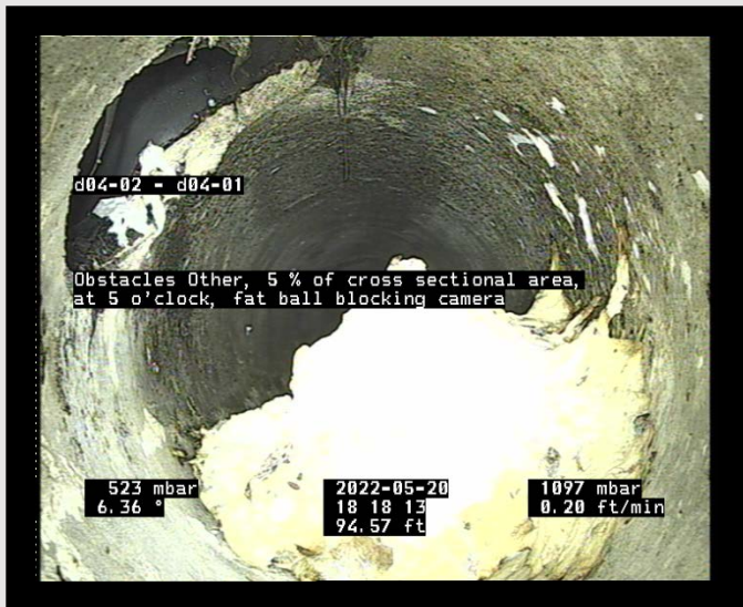
Picture of grease glob in sewer mainline.
