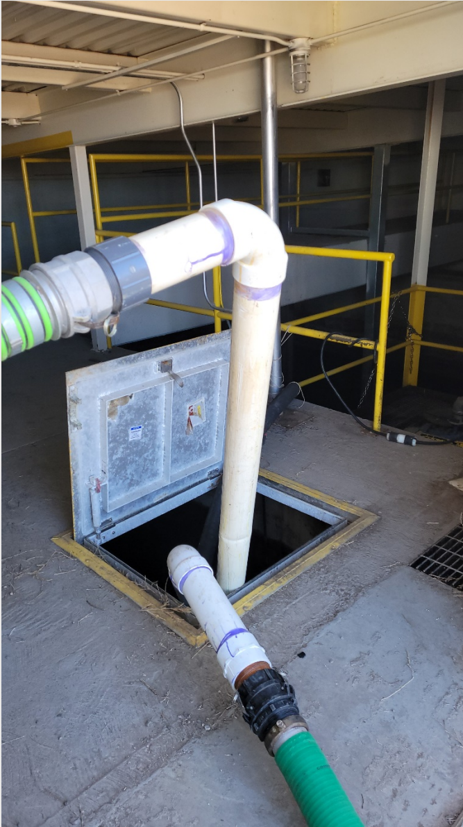
Overflow Basin at Wagon Wheel Lift Station
