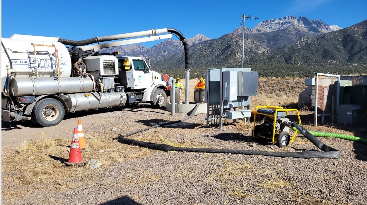
Manual wastewater pumping operation at Wagon Wheel Lift Station
