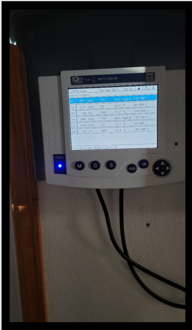
Picture of new monitoring equipment display At Aspen WWTP
