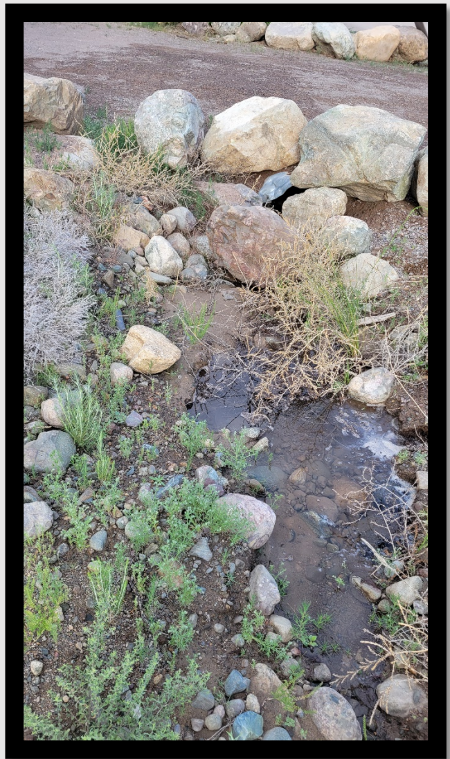
Pictures of water main break at 2212 Spanish Creek Way.
